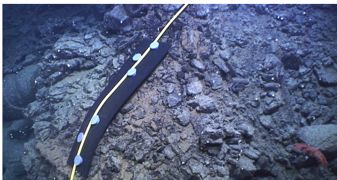
We installed rubber mats to protect the observatory extension cable at stress points where the cable is draped over sharp rocks and deep crevasses. 2110m depth
